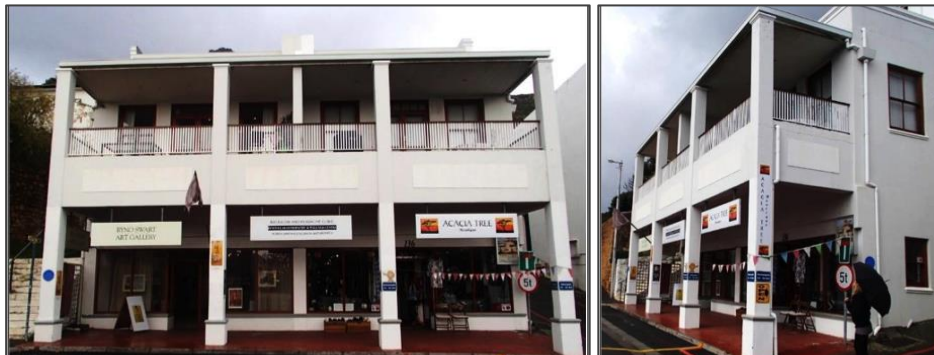
Figure 1: (Left) The street view of Malawi House, Simon's Town showing the encroaching balcony and pillars. Right: A side view of Malawi House, Simon's Town. (Photographs: L Humby 26/06/2014)
